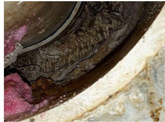
Image 28: Asbestos rope in floor penetration
