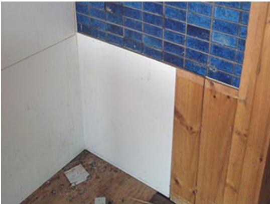
Image 3: Asbestos sheeting under tiles
