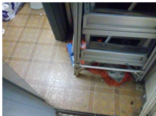
Image 27: Asbestos vinyl sheeting
