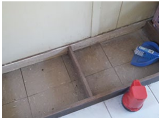
Image 20: Asbestos tiles and blackjack glue hidden under built in furniture
