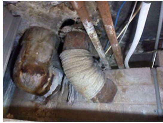
Image 40: Pipe sound insulation
