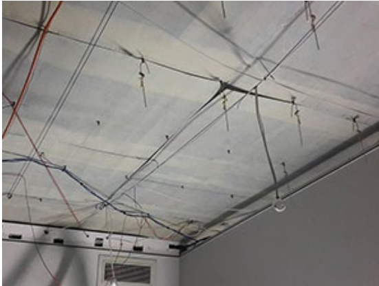
Image 11: Asbestos coating under ceiling
