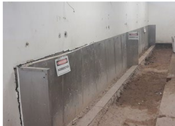
Image 22: Asbestos backing on urinal
