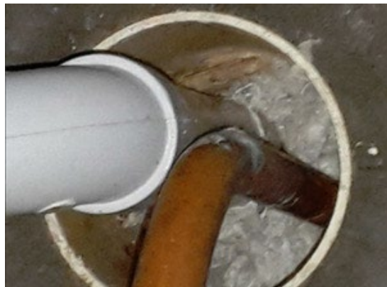
Image 29: Asbestos rope in floor penetration
