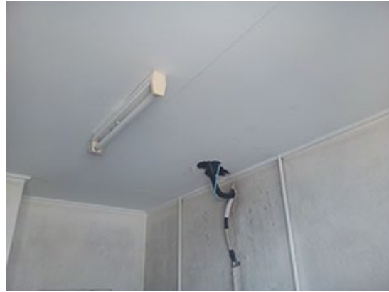
Image 24: Asbestos ceiling panel
