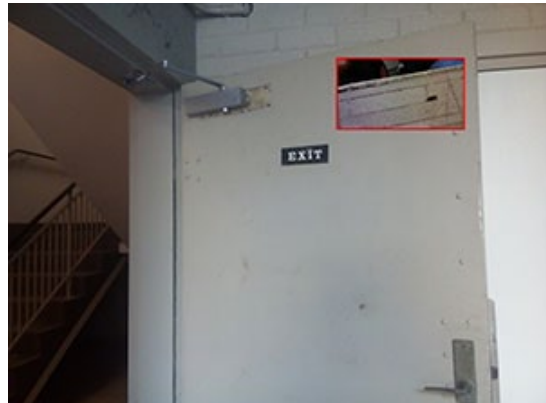
Image 36: Asbestos within fire door
