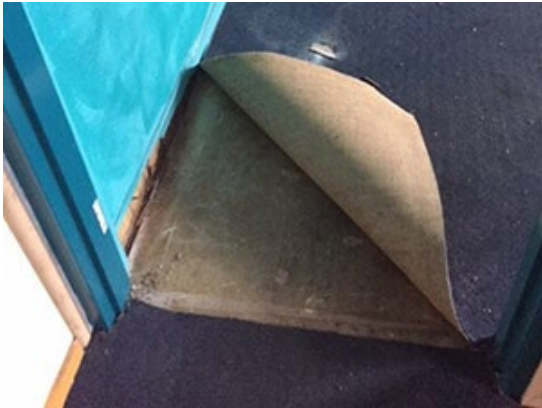
Image 7: Asbestos paper underlay
