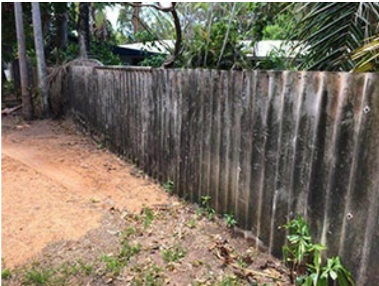
Image 17: Asbestos super six fencing
