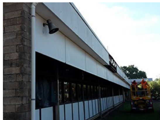
Image 26: Asbestos panels and eaves
