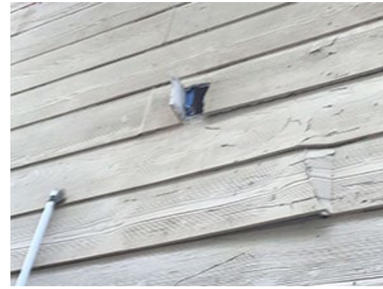
Image 12: Asbestos wall cladding
