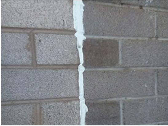
Image 15: Asbestos joint gap sealer
