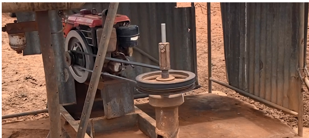
Image 1: The pump's moving pulleys and belt unguarded, are a hazard for nearby workers. (Source: NT Police)
