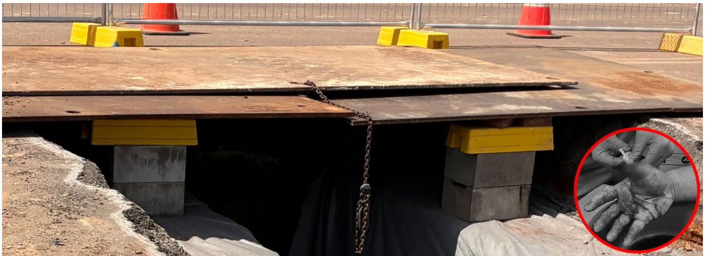
Image: The incident site showing the trench plates being held up by improvised dunnage. (Insert) The worker receiving medical treatment for their injury.
