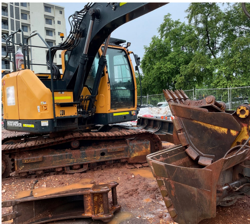
Image: The excavator and buckets in situ after the incident.
