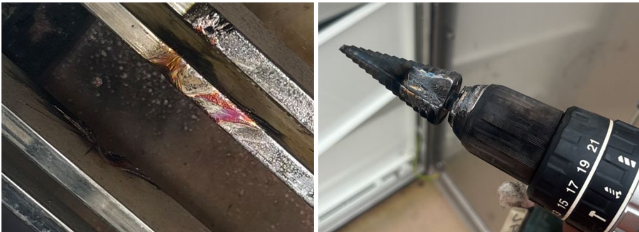
Image 1: (Left) Damaged busbar after contact with the drill bit. (Right) The step drill showing oxidation and discoloration.
