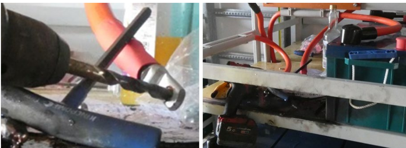
Image 2: (Left) Cable lug being drilled out. (Right) The cable was still attached to the battery.
