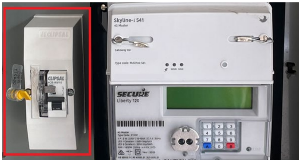
Image. New style electronic meter with circuit breaker as a meter isolator, highlighted in red.
