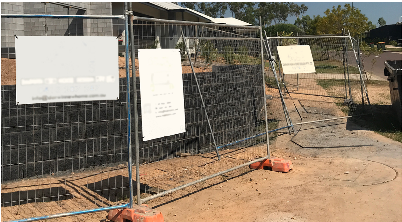
Image 1: The effectiveness of this temporary fence in preventing access is questionable. (Source: NT WorkSafe)
